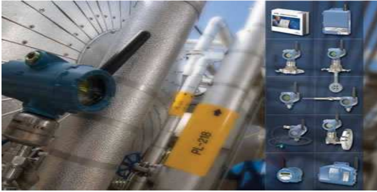
Figure 2: Wireless temperature transmitter of BP's Cherry Point plant [11], Emerson process management ( http://www.emersonprocess.com ).
